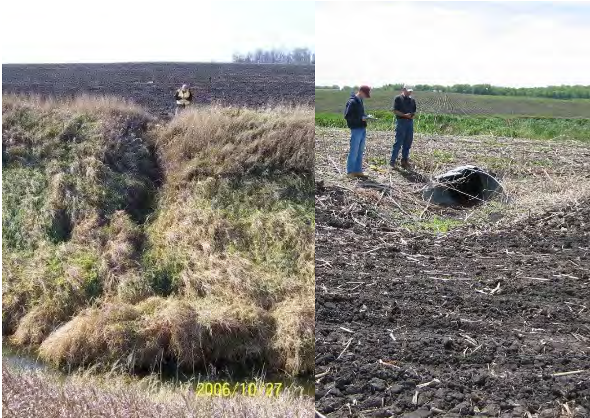
Fig. 2.1 Example photos of a gully (left) and a side inlet (right) in the field
