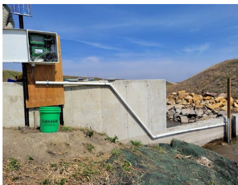
Martin County ditch #28 nutrient treatment wetland outlet weir structure
