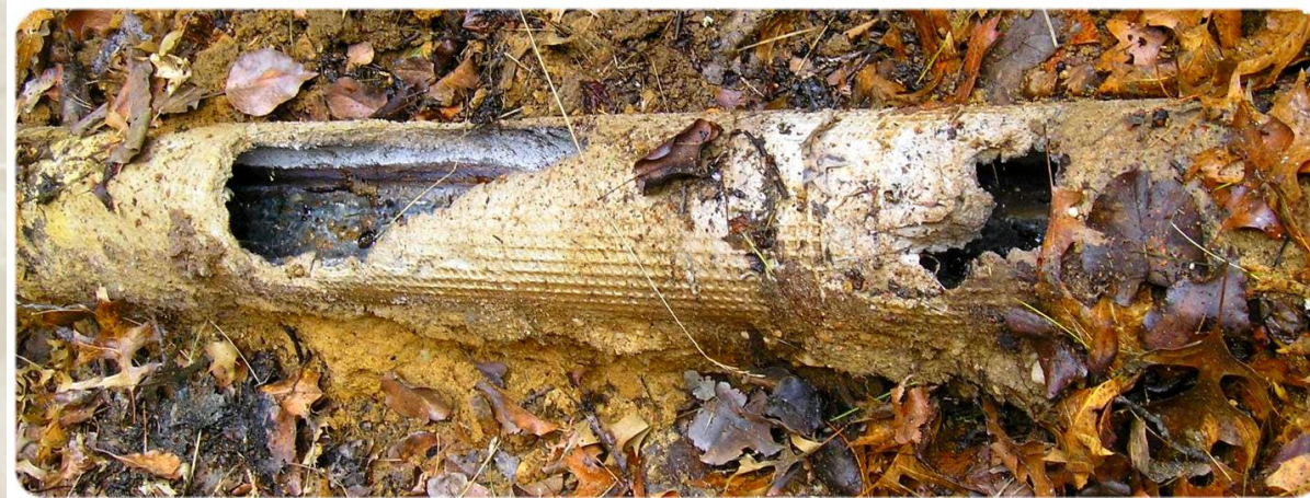
Orangeburg pipe (1950-1972) wood fibers & tar
