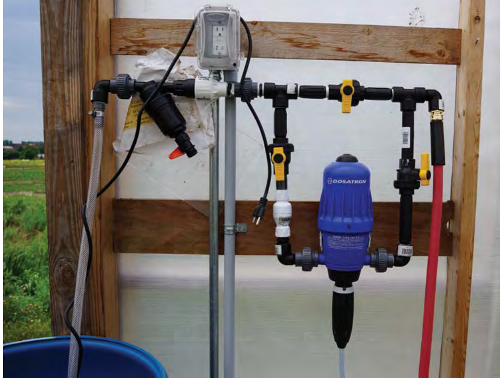
Dosatron assembly for fertigation at The Good Acre.
