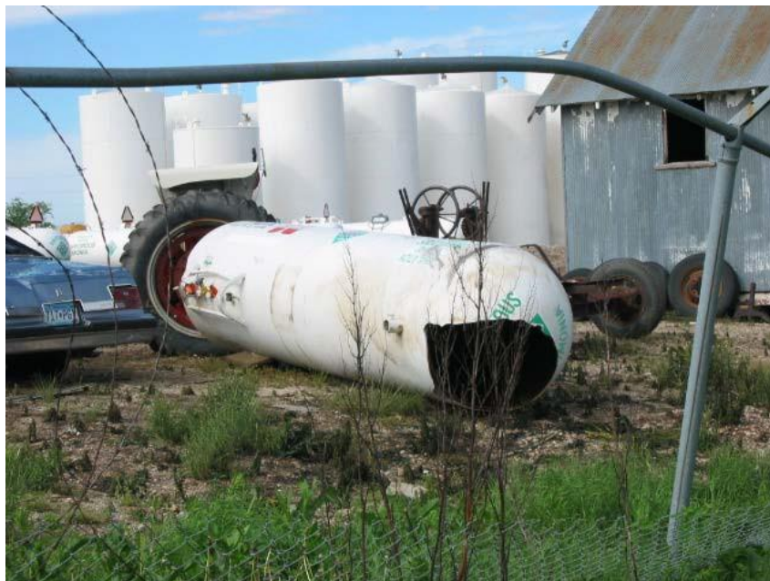
Large opening where the tank failed. Absent shell piece remained by load out risers.
