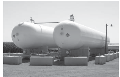
Anchored/stabilized concrete barriers with access gaps of no more than 3 feet. Warning markers to a height of 3 feet are required for barriers that are less than 3 feet in height.
