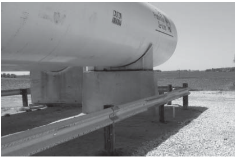
DOT approved guardrail attached to posts at a height of at least 3 feet. Each post is positioned every 10 feet and is anchored into the ground by a 12 X 48 inch concrete foundation.
