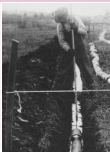
Tiling was hard work in the early 1900s. Clay or concrete tile was laid less than 3/8' apart on a slight slope. The opening between tiles allowed for water to slowly move out of the soil and into the tile. The slope sent it off the field and into a drainage ditch. Farmers could then plant crops such as corn, wheat and oats.
