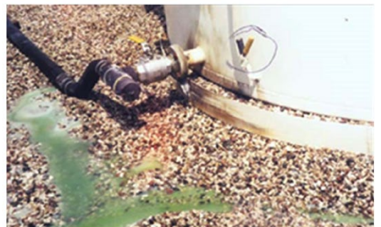
A leaky fitting caused pooling of fertilizer in a rock bed
