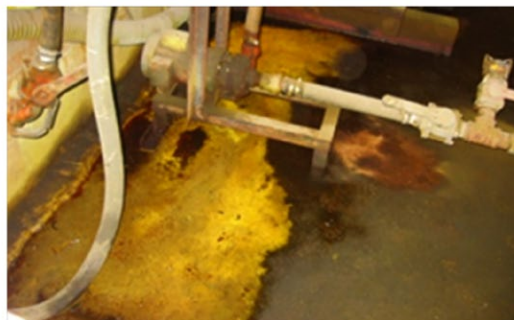
Unaddressed pesticide spills can compromise dike integrity
